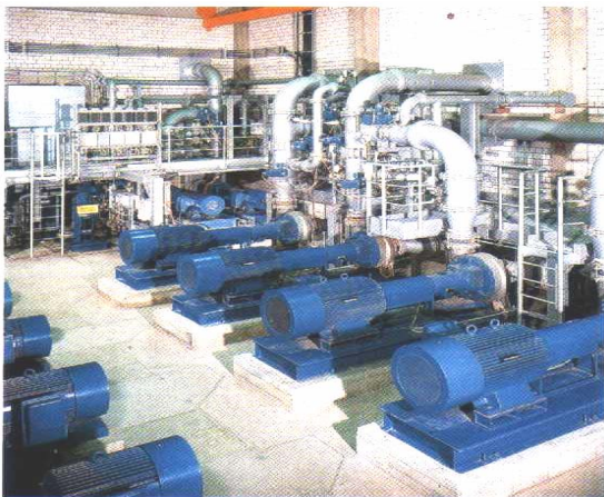
Figure 11: SCHORCH Motors 160KW, 400V, 1485rpm, Driving pumps
