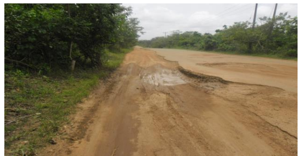
Plate 2: Abandoned Road Project in Ajagba Village in Iwo Local Government Area.
