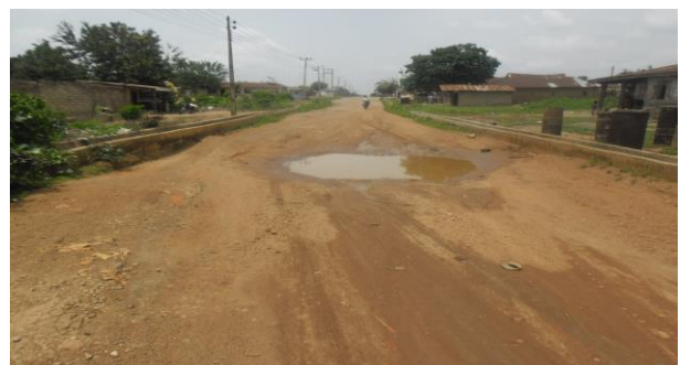
Plate 3: Abandoned Road Project in Ilawo Town in Ejigbo Local Government Area.
