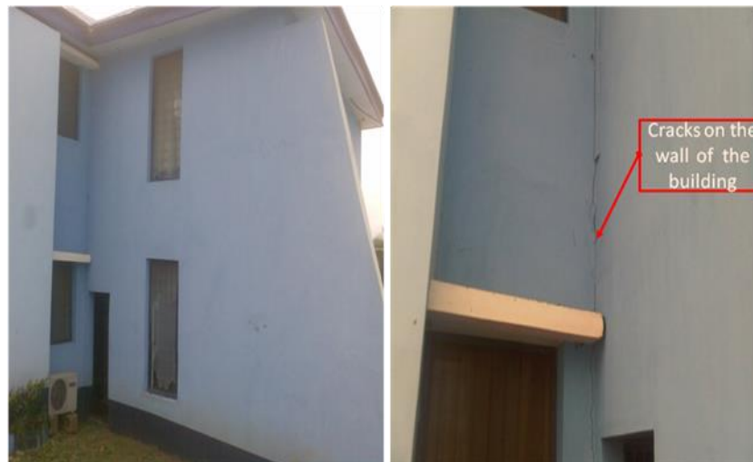
Figure 1: Crack from First to the Ground Floor of the Story Building.
