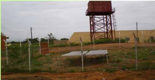
Solar Water Pumping for Students in Sokoto, Sokoto State
