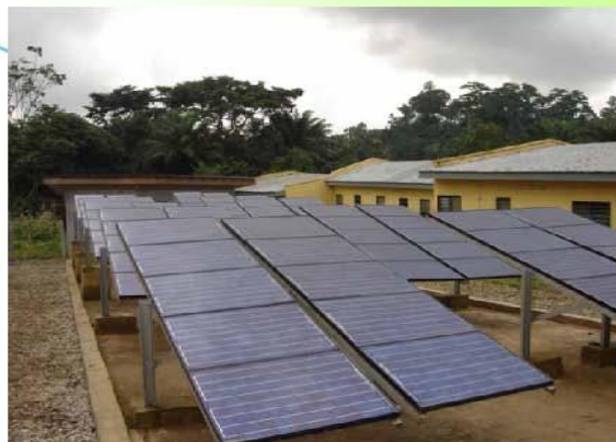
Solar PV at Ilaje, Ondo State of Nigeria
