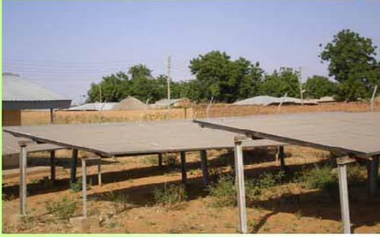
Solar PV mini-grid in a village in Sokoto, Sokoto State
