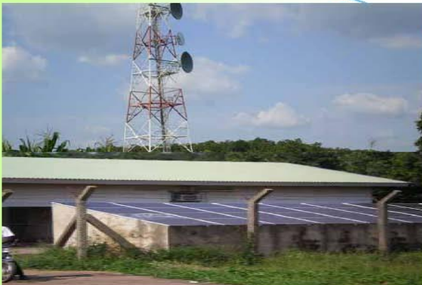
Solar PV for Telecommunication 20km Kaduna-Abuja Road
