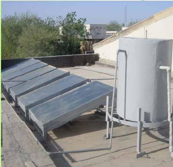
Pilot Water Heater at UDUTH by SERC, Sokoto
