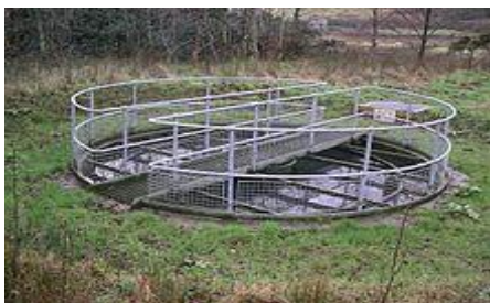
Figure 6: Secondary sedimentation tank at a rural treatment plant.
