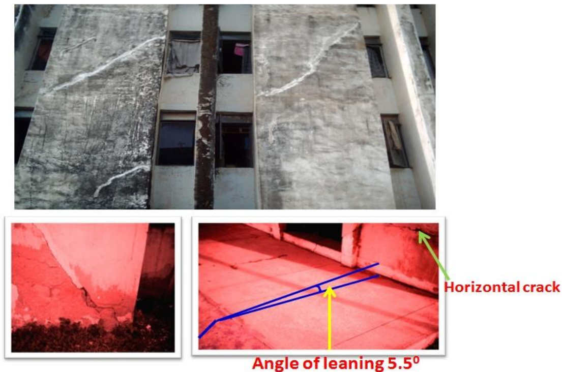
Figure 3: Danger of Diagonal Cracks, Horizontal Cracks, and Angle of Leaning (Site 3).
