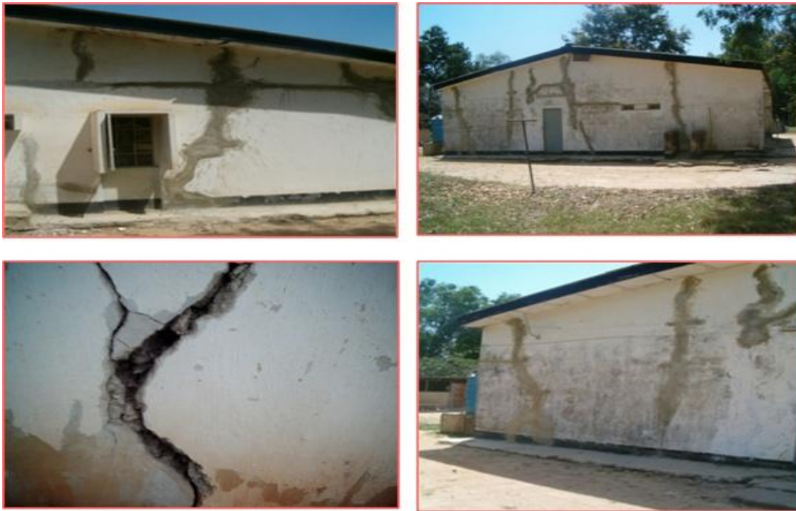
Figure 2: View of Some Cracks on Site 2 Building.
