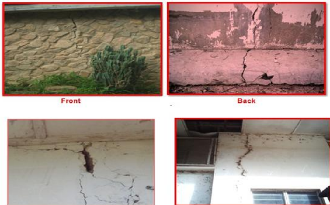
Figure 1: Some Views of Cracks on Site 1 Building.
