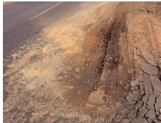
Plate 1: Typical Failure Pattern.
