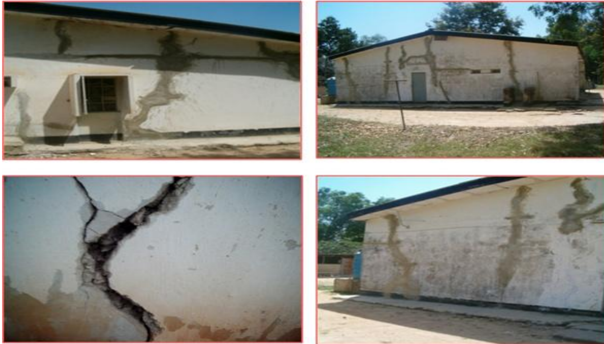
Figure 1: Some Views of Cracks on one of the Buildings (Site 2).
