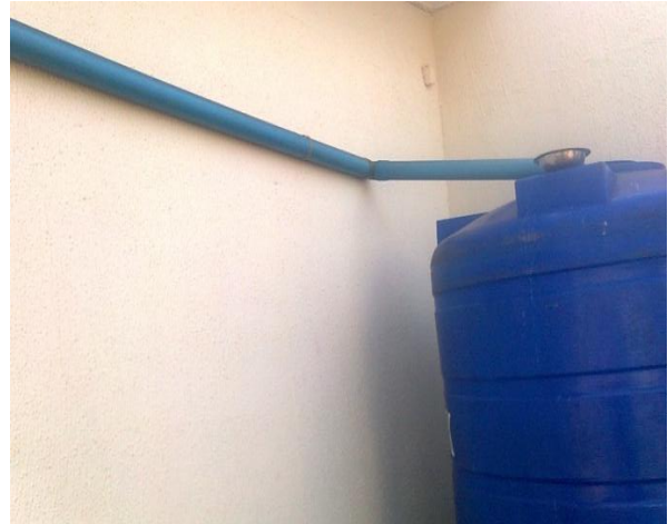
Figure 5: The Channel Leading to the Storage Tank.
