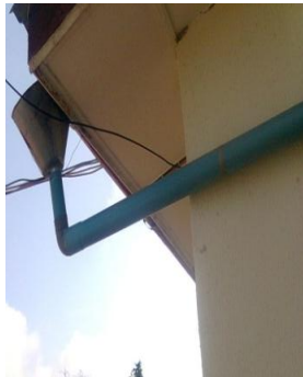
Figure 3b: The Funnel and the PVC Pipe Conveying the Water to the Storage Tank.
