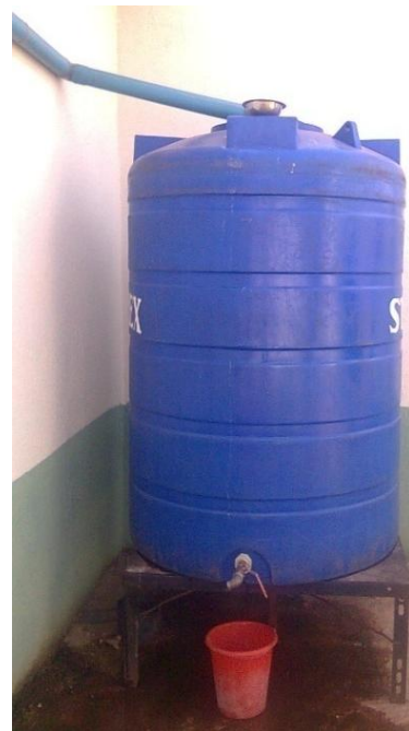
Figure 6: The Channel Leading to the Storage Tank.
