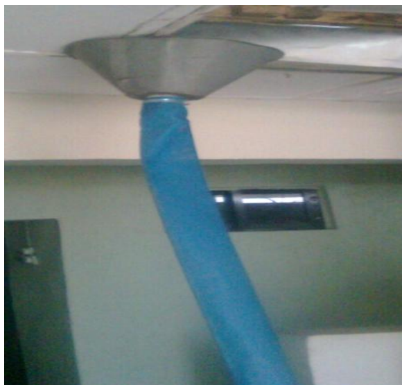
Figure 7a: The Second Drain for Initial Water Run-Off.
