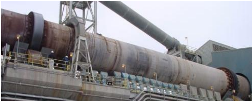
Figure 4: Cement Manufacturing Plant Clinker Producing Kiln.
