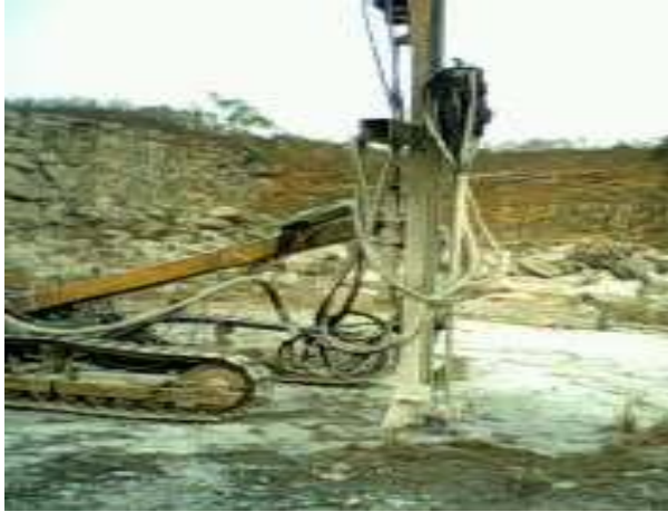
Figure 5: A Photograph Showing a Hydraulic Drilling Machine used to Drill Holes down the Crustal Layers during the Rock Blasting Process in Quarries.
