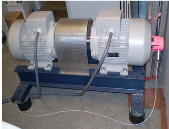
Figure 2: Photograph of the 7.5kW CHP Induction Generator.
